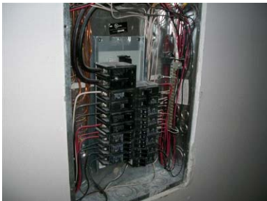
Main 100 amp panel
