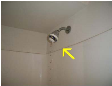
Leakage at shower
