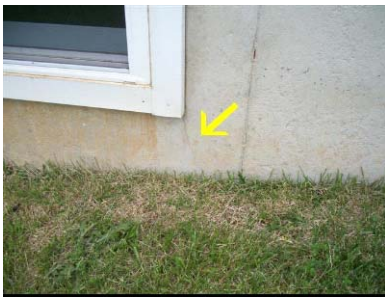
Crack at rear
