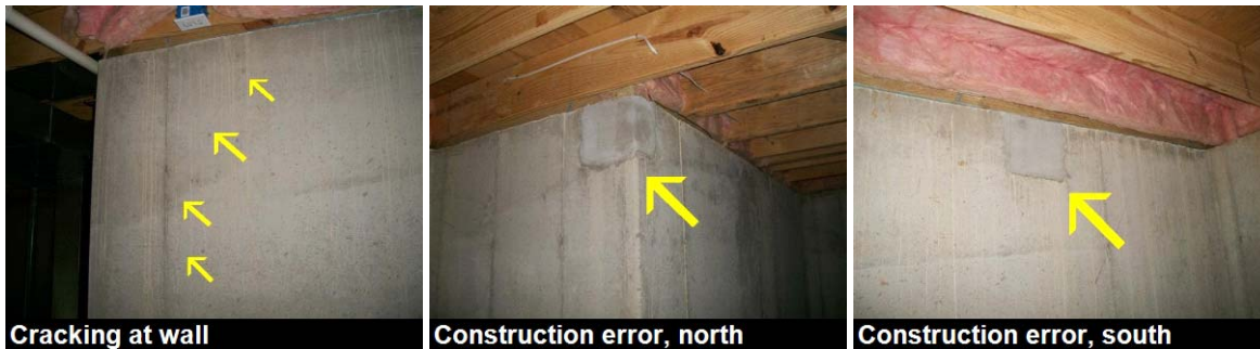
Cracking at wall
