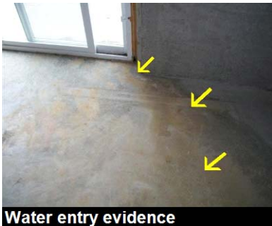
Water entry evidence
